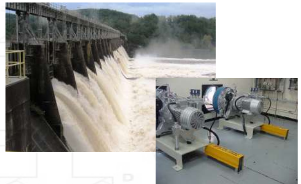
Compress Air Supply & Steering of Pneumatic Operated High Voltage Switch in Hydro Dam
