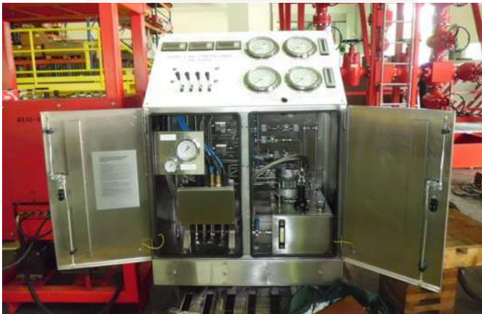
▲ Choke & Kill Control System
